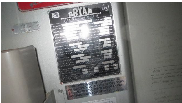
Boiler name plate.
