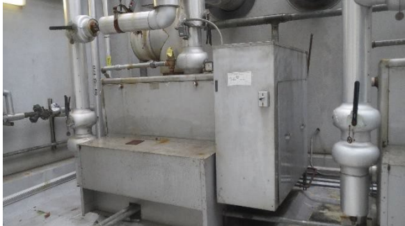
View of boiler B-1.
