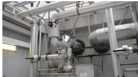
View of boiler gas vent through wall.
