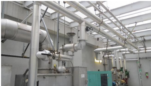
View of 18" gas vent duct.
