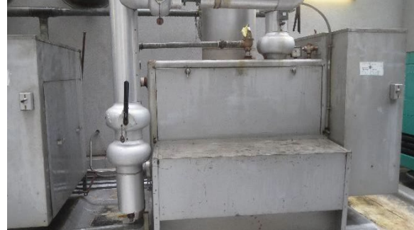
View of boiler B-2.
